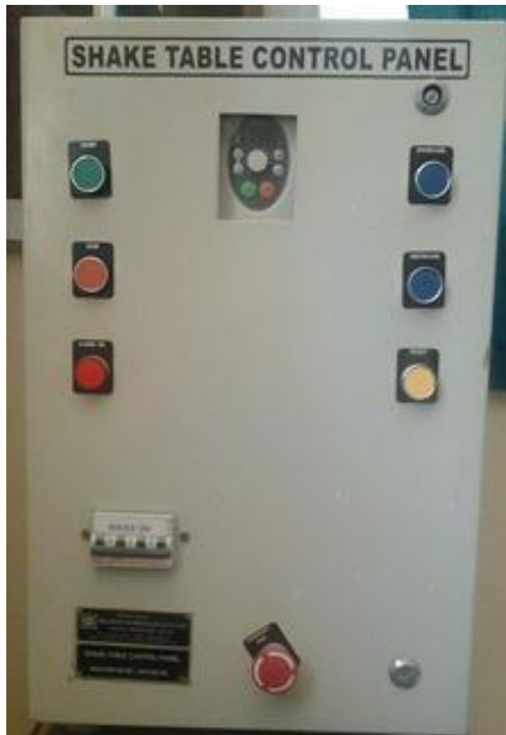
3. Figure3.4: Control Panel
